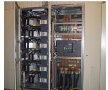
Six of the 40 capacitor steps besides the 5,000 A CB
