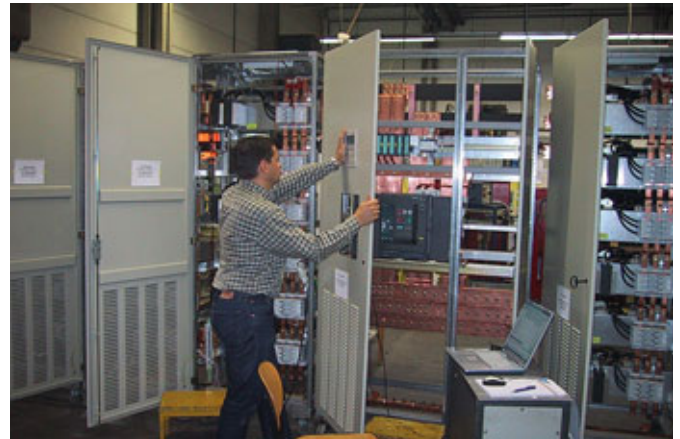
Factory tests of the PLC-programming
