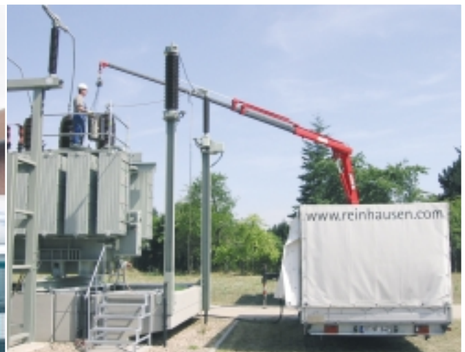
Rolling workshop with crane wagon Crane: Range: 13.60 m, load at max. range: 320 kg
