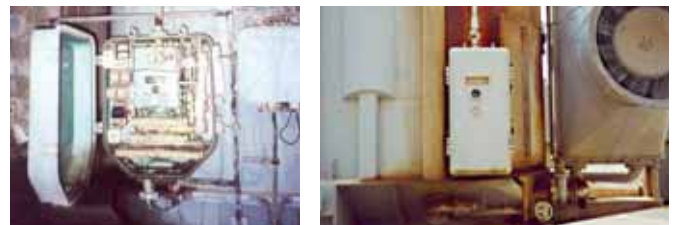
Photos show the installed OLTCs in the 70 MVA and 20 MVA TUR transformers at PEEGT Syria.
