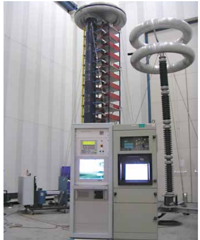
Fig 4: Control and measuring system at KEMA/The Netherlands
