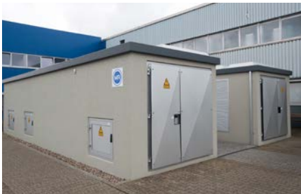
The 2 dynamic systems supplied in the form of concrete stations for safety reasons.
