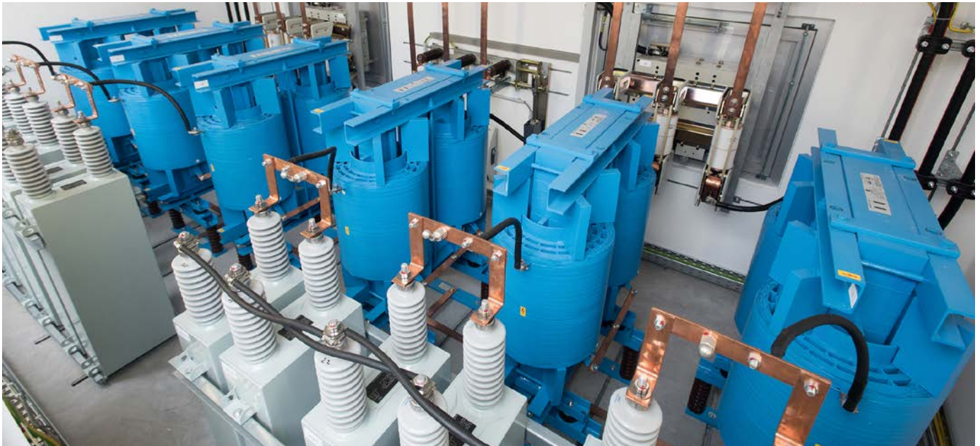
View into the MV part of the hybrid system with restrictors (blue) and MV capacitors in the foreground.
