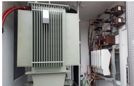
Step-up transformer to increase the voltage from 690 V to 30 kV for the dynamic part of the system.
