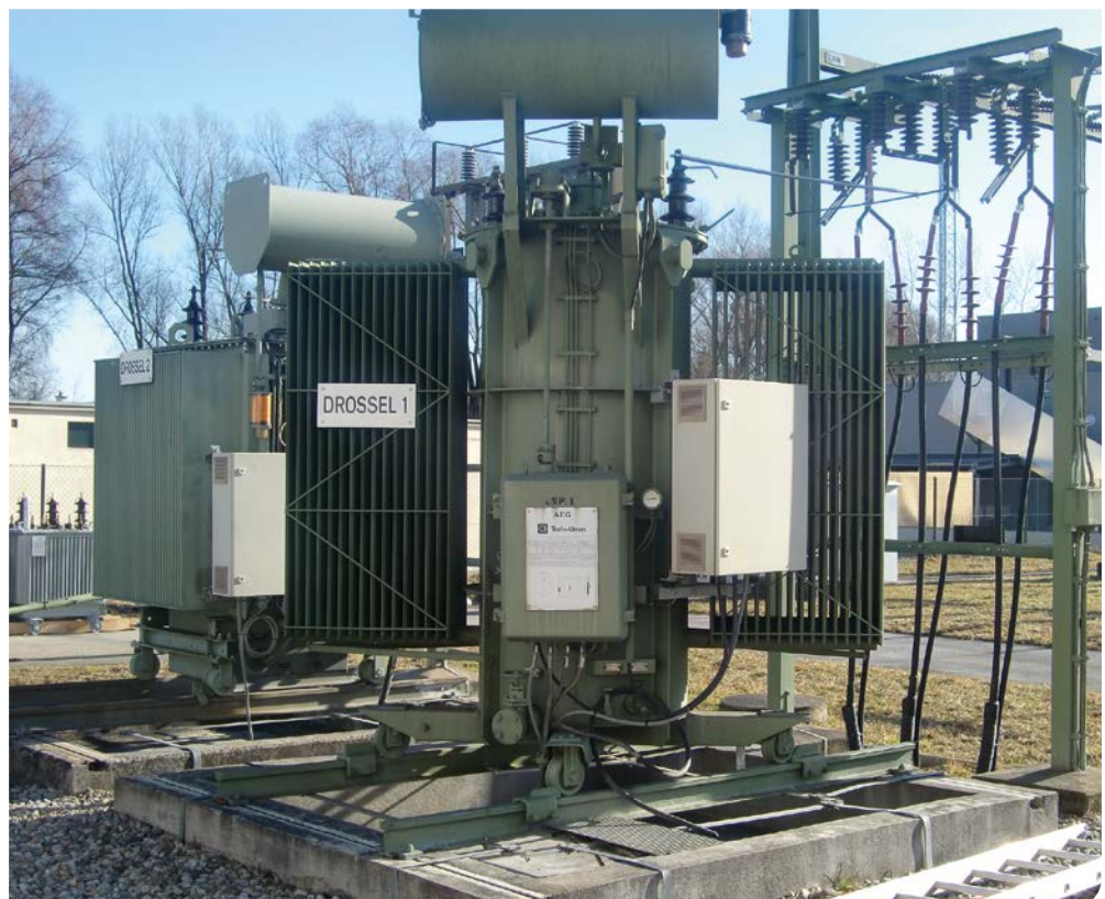
Arc suppression coil (Petersen coil) with AEG motor-drive unit before replacement.
