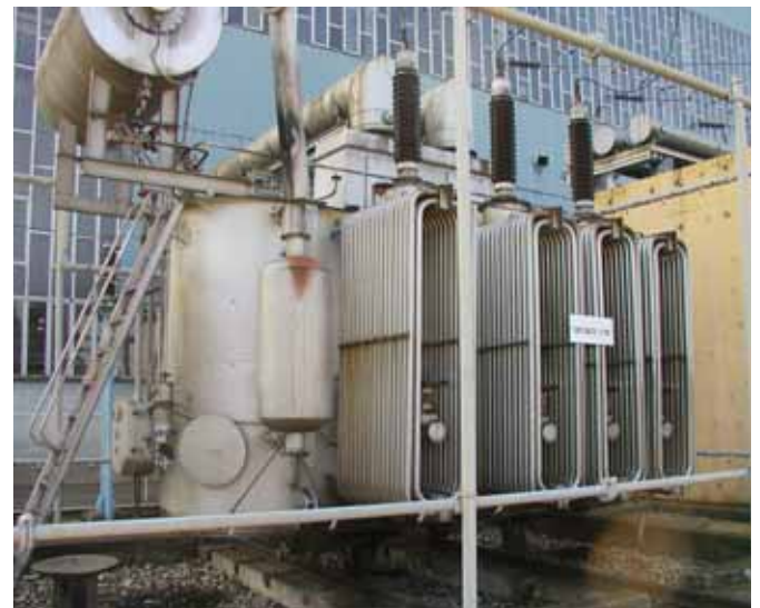
28 years old transformer
