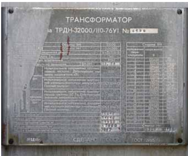
Type plate of the transformer
