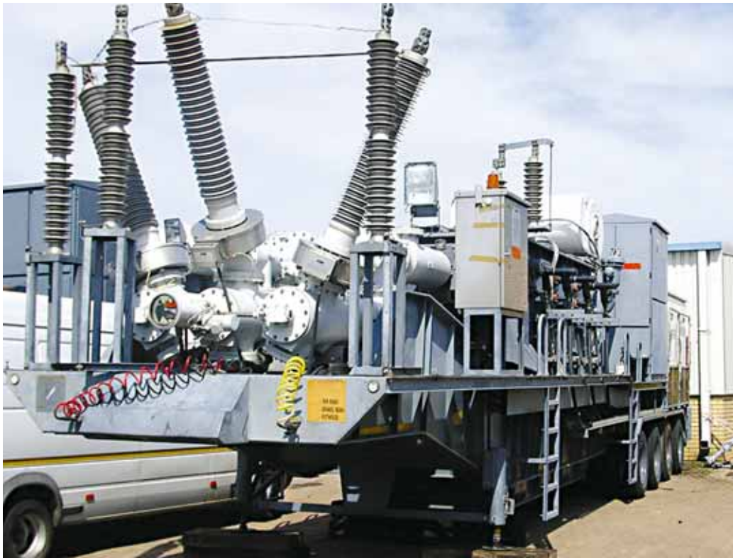
The "Ubejane" Mobile Transformer of Eskom Pietermaritzburg retrofitted with Messko instruments.
